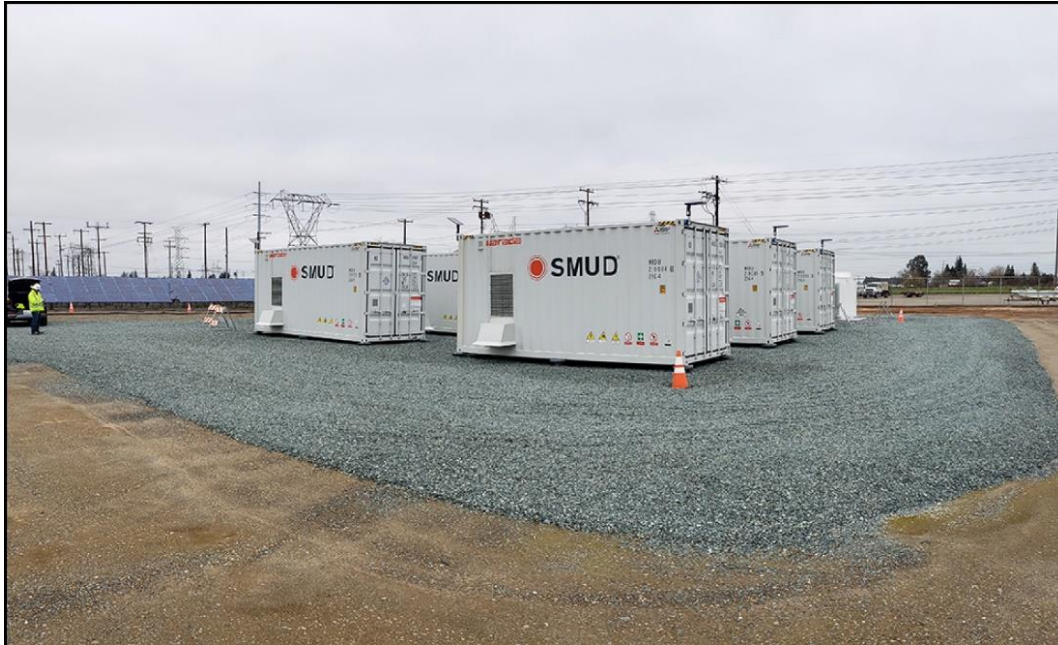
Exhibit 2-6. Battery Energy Storage System
